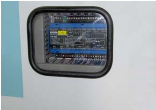
Y19 Example of window in door for viewing internal components
