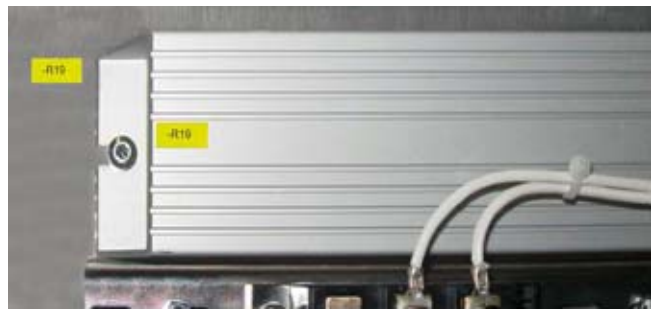
M96 Example of dual marking of items of equipment
